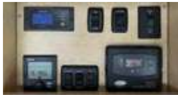
Convenient control center monitors capacities
