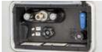
Water and utility management center
